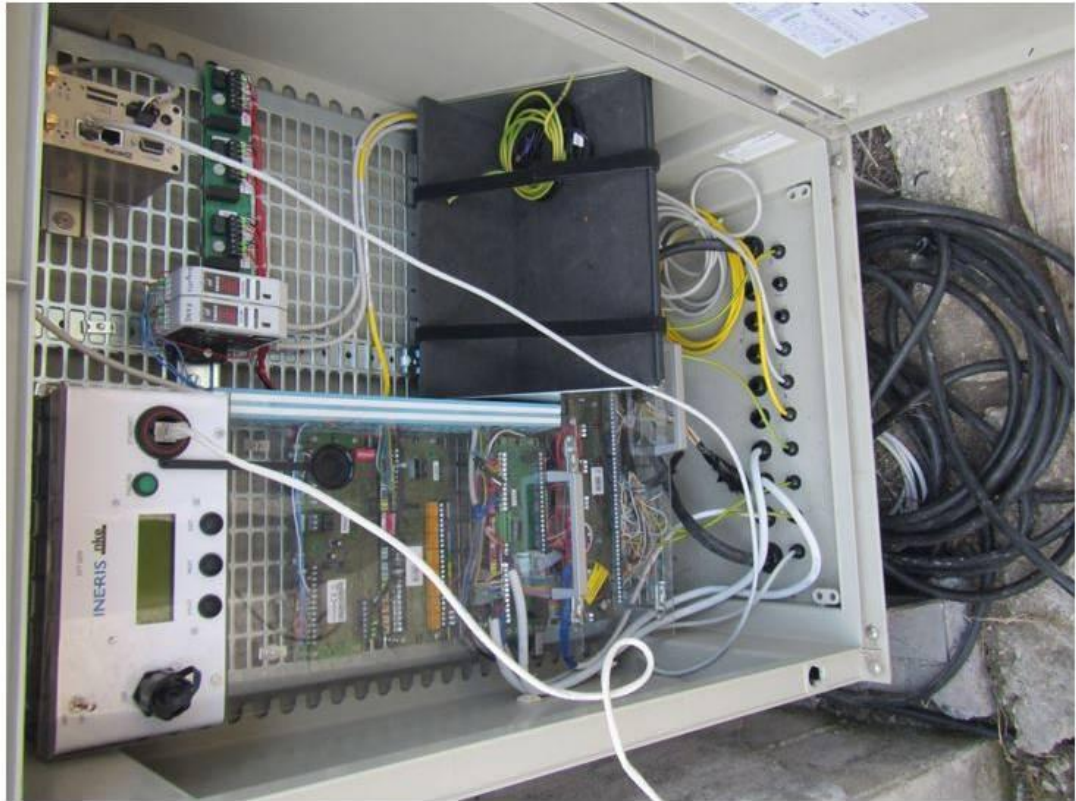
DataLogger – Farm Station
